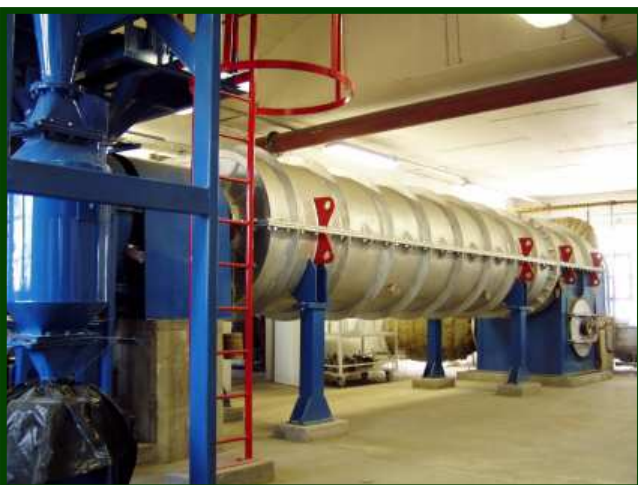
3R CARBONIZATION EQUIPMENT
